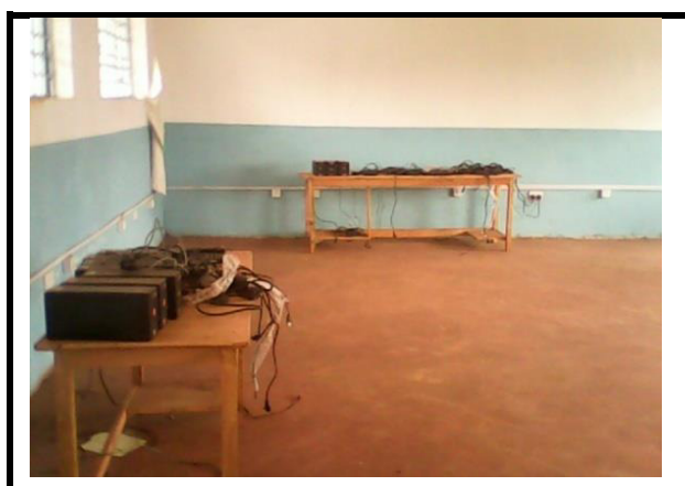
Photograph 4.2: A photograph showing a vandalized computer lab
