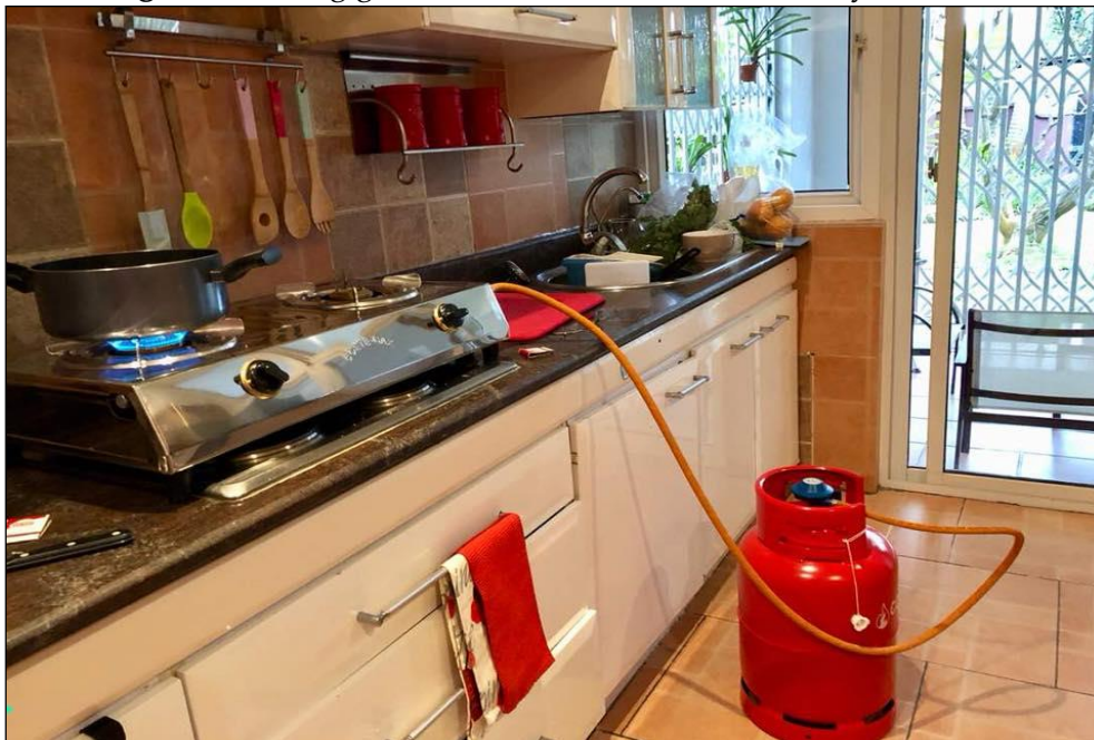
Figure 5: 12.5 kg gas bottle connected to the stove by the hose
